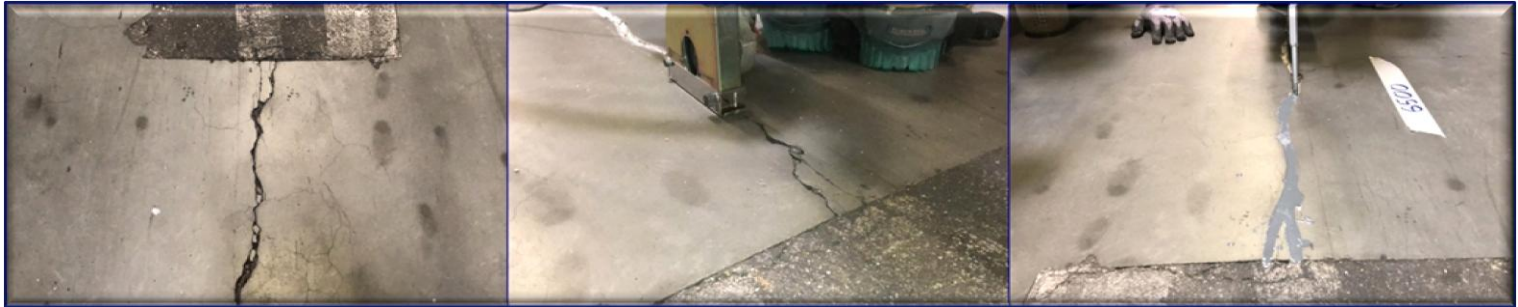
Cracks in the concrete
